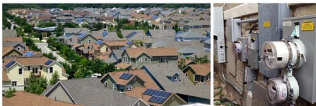
Fig. 1. Left: Mueller homes equipped with rooftop PVs (6 kW each). Right: Second (research) meter in a dual socket configuration. (Image source: Pecan Street, Inc.)
