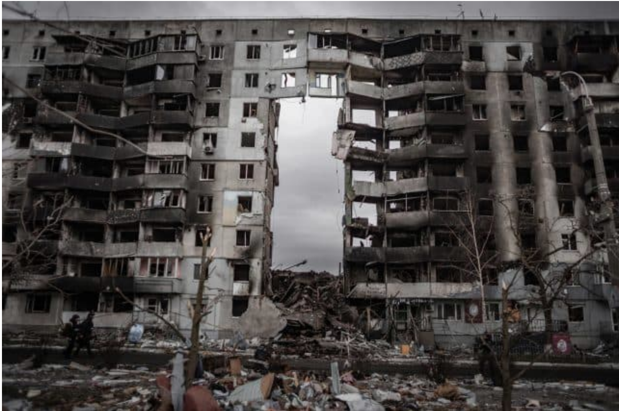
A ruined apartment building in Borodianka, Ukraine, on April 6, 2022. Russian armed forces bombarded the town during their assault on Kiev in March. Source: Pexels .
