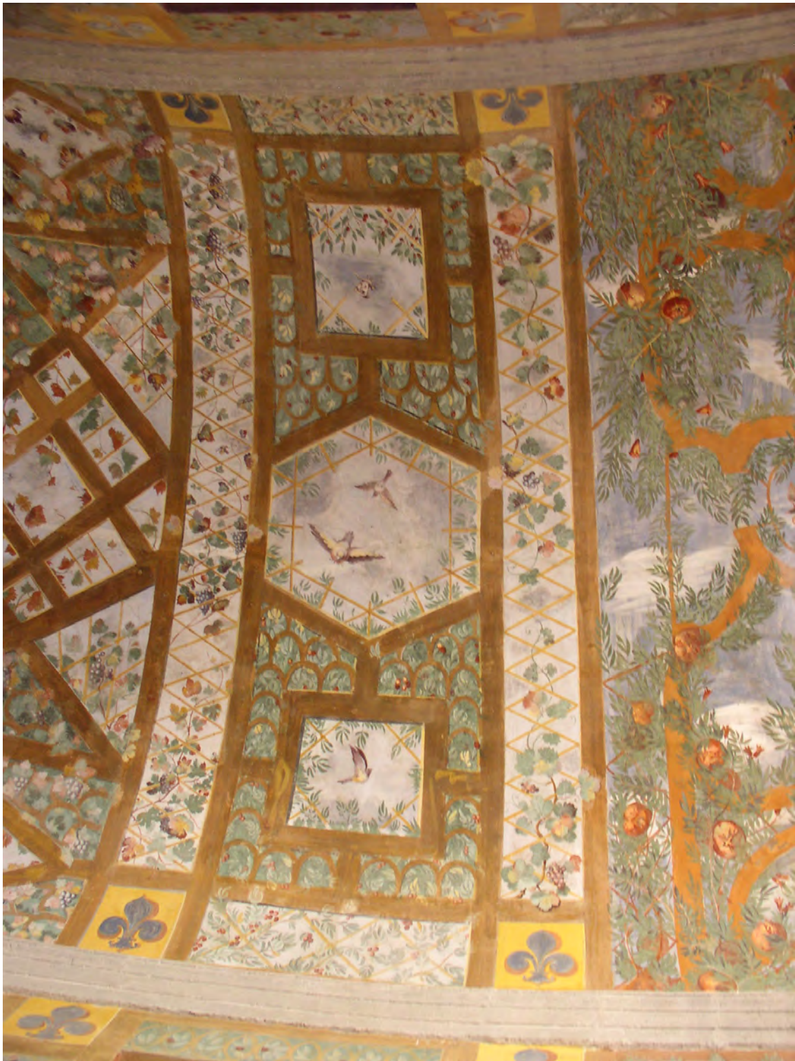
Fig. 6.66 Villa Farnese at Caprarola, circular portico, illusionistic pergola, section 9N (photo: author).
