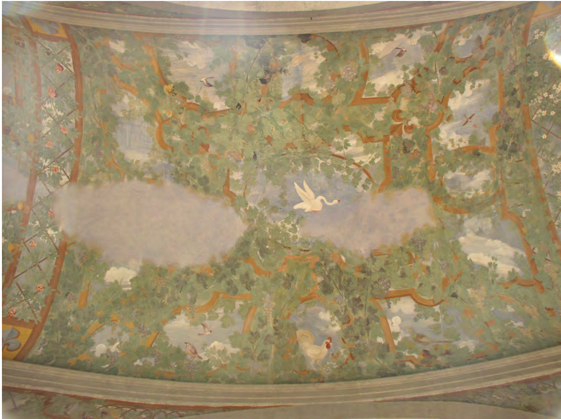
Fig. 6.61 Villa Farnese at Caprarola, circular portico, illusionistic pergola, section 7W (photo: author).
