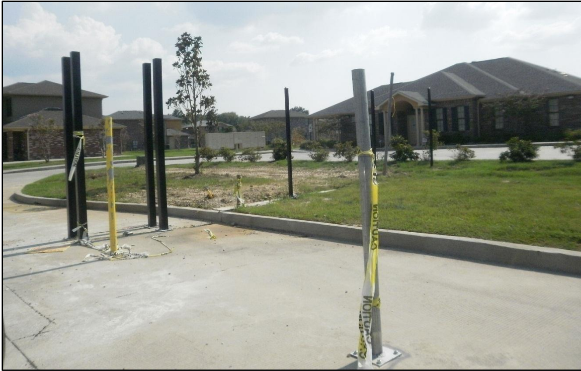
Figure 17: Gate under construction at Townhomes of Sherwood Forest. Leasing office at right; townhome at left.
