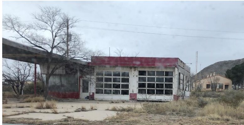
Photo 3: One of many abandoned gas stations in Sierra Blanca. Source: Scott Winton
