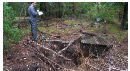
Figure 3. (a) Brian Cowan, geologist for Zara Environmental documenting Sinky Dinky Cave in 2012. Unstable sediment collapsed into the 20-foot-deep cave presenting a public safety threat. (b) Sinky Dinky Cave in October 2014 after restoration, but prior to landscape revegetation
