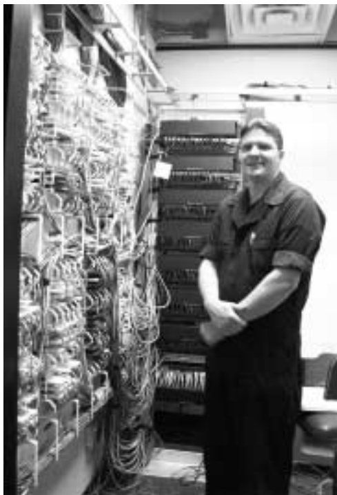
Network Analyst, Jason Dendy, in one of five Welch Hall wiring closets
