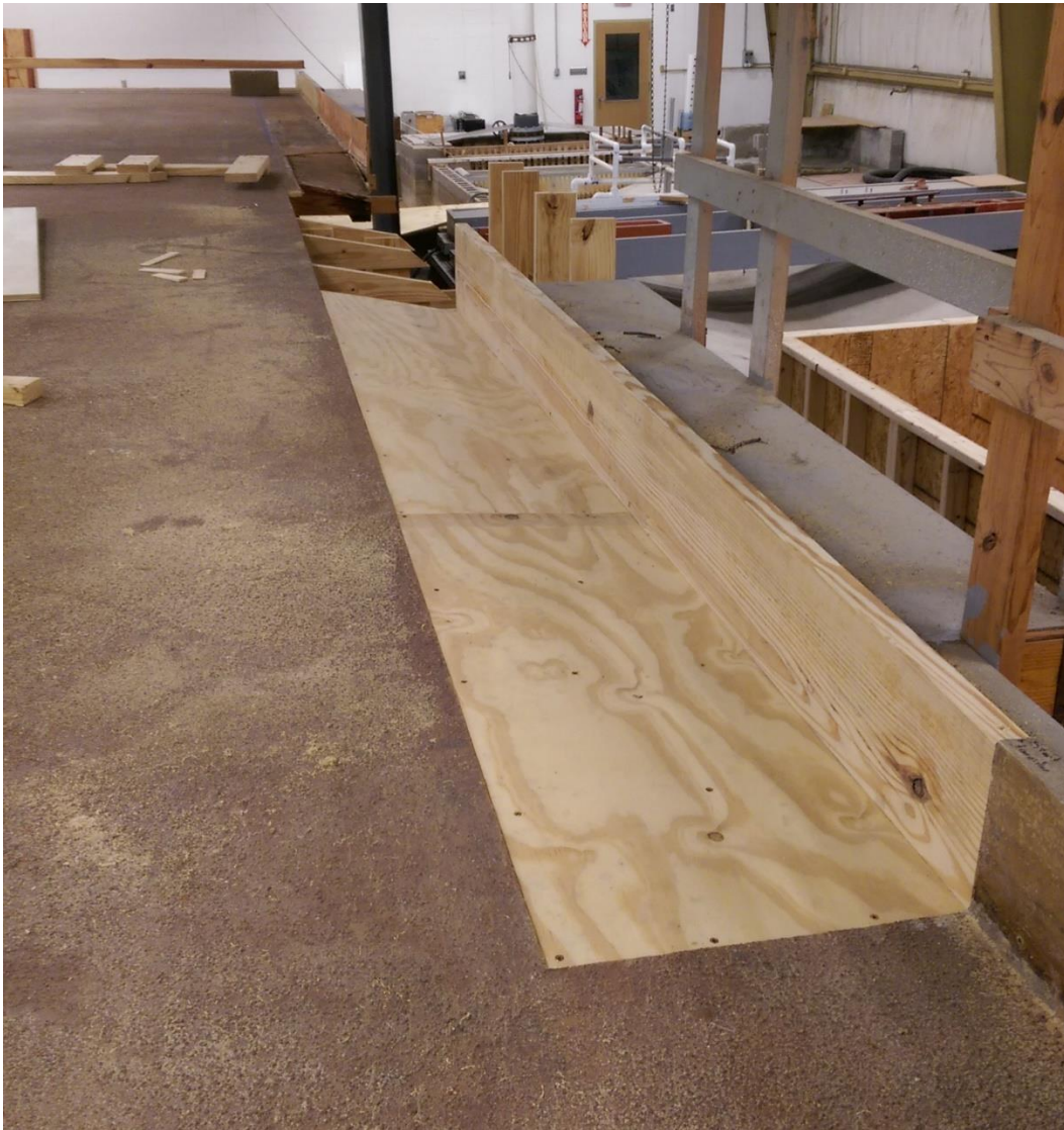
Figure 54. Photo of upstream curb and gutter transition under construction and before texture is applied.
