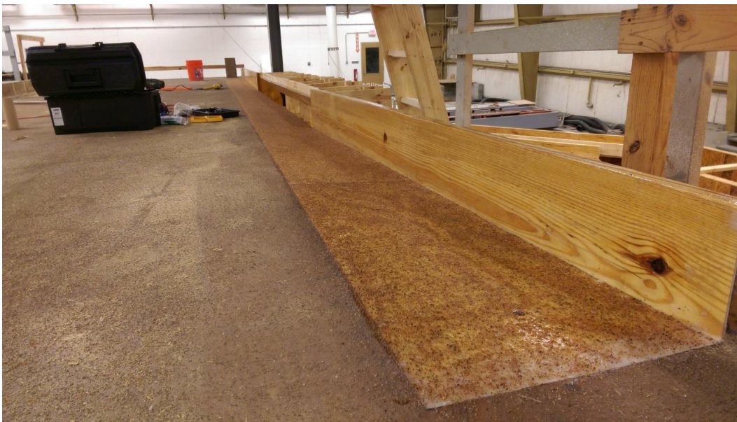
Figure 15. Upstream curb and gutter transition and TxDOT curb inlet.
