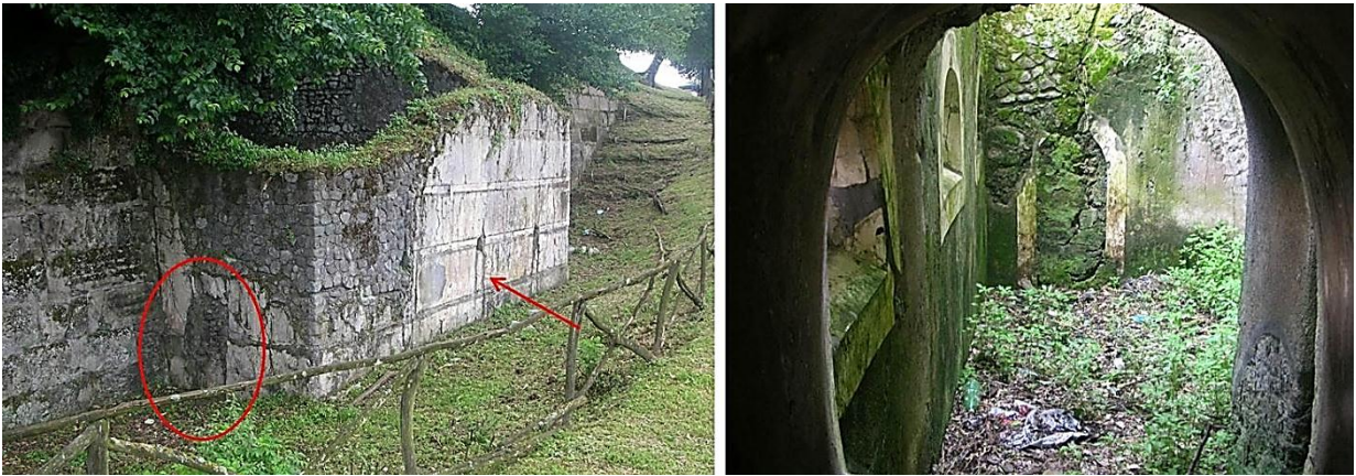
Figure 89 Tower VIII. Left: Note the walled up postern and modified arrow slits, right: White stucco frames on the interior, photo author.
