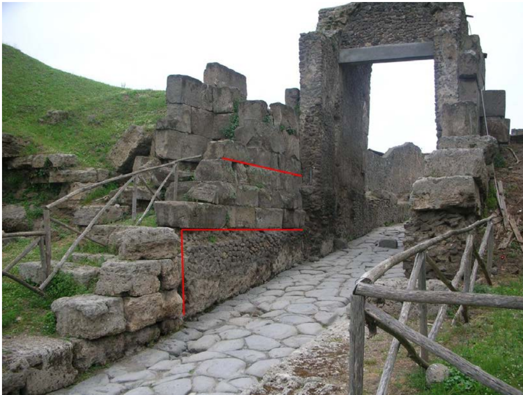
Figure 43 The Porta Nocera and its exposed foundations. The red lines indicate the concrete and the exposed tufa foundation blocks, photo author.
