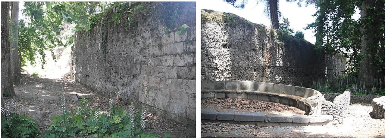
Figure 69 The opus incertum sections on either side of the Porta Stabia, photos author.
