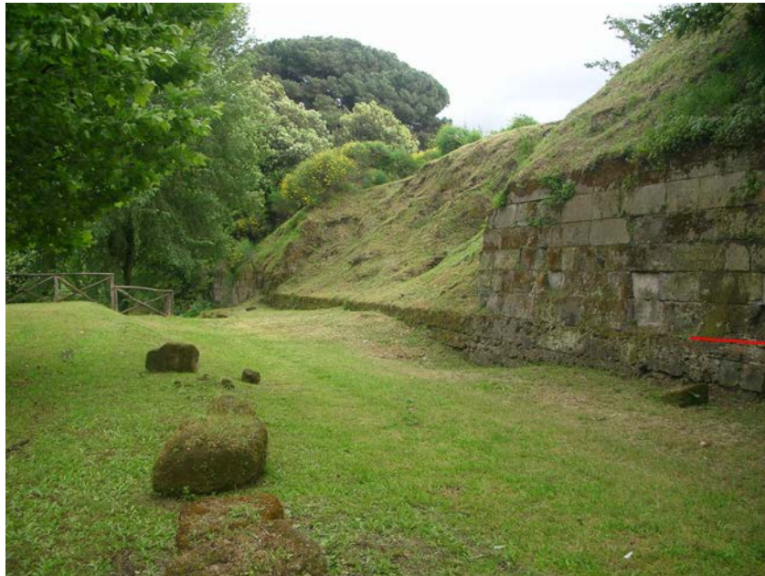
Figure 38 Curtain wall near Porta Nola. Note the red line indicating the switch between limestone and tufa. The large section of missing tufa masonry was likely looted after the earthquake, photo author.
