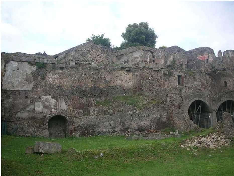
Figure 73 Section of the city walls east of the Temple of Venus, photo author.
