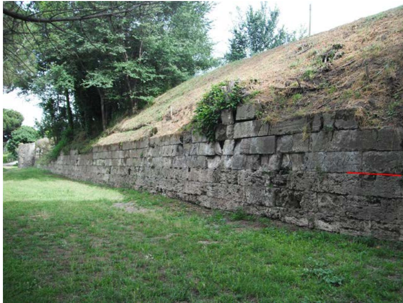
Figure 37 Wall curtain near Tower VII. The red line indicates the separation between limestone and tufa, photo author.
