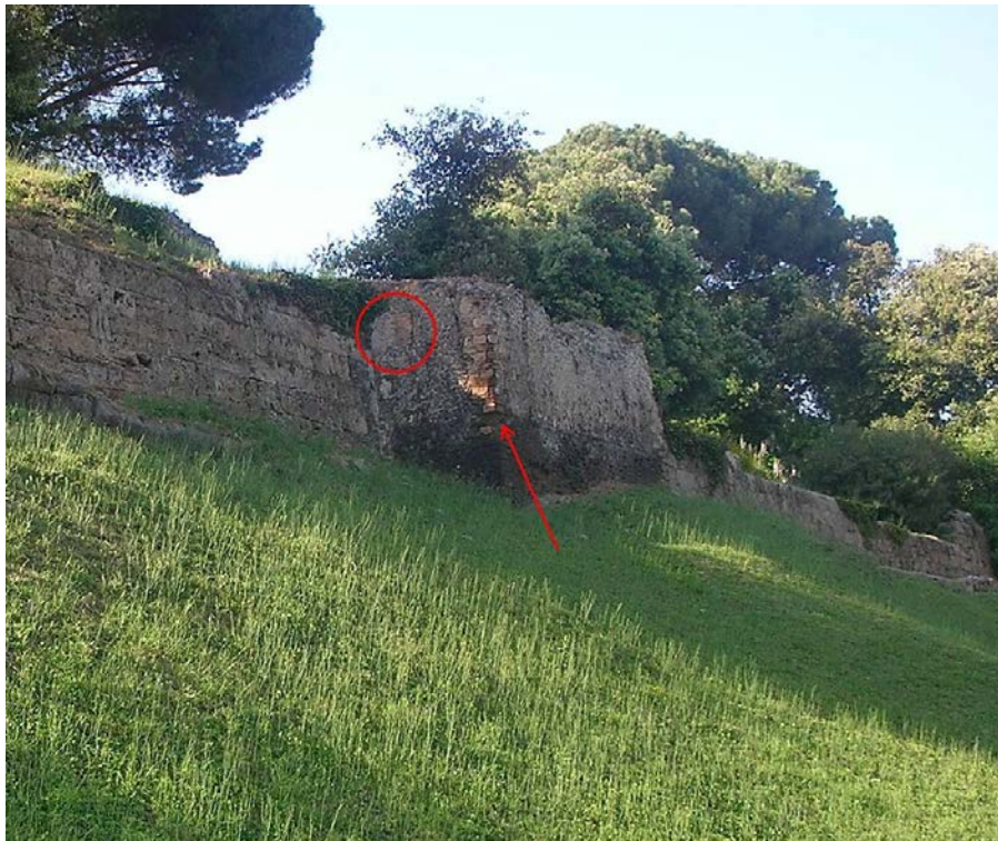
Figure 85 Tower III. The red circle denotes the brick patchwork. The arrow indicates the quoin repairs and the line of exposed foundations, photo author.
