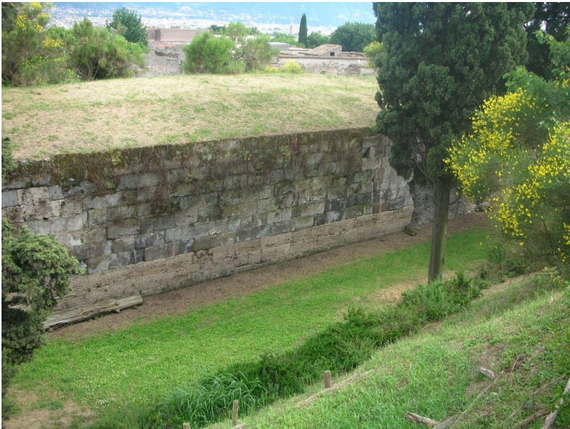
Figure 32 Wall curtain between Towers XI and XII highlighting the differentiation between limestone and tufa, photo author.
