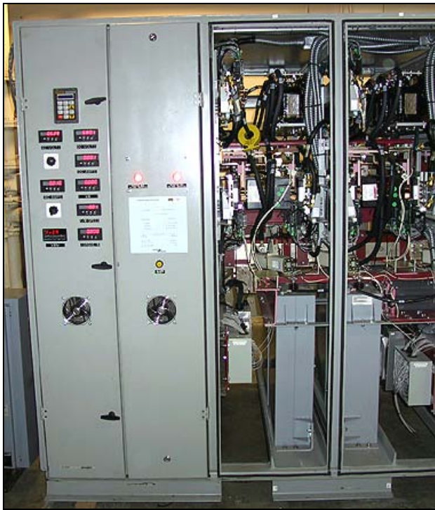
Figure 2: Operational ARCP converter showing control bay (left), brake bay, and the A & B phase bays (right, doors off).
