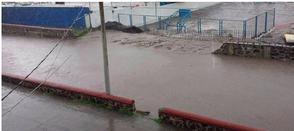
Figure A-4: Ruptured Drainage Channel (Source: Evalúan daños)
