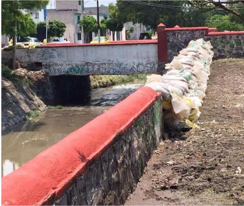
Figure A-3: Ruptured Retention Wall on Río Querétaro (Source: Torres & Benítez 2014)
