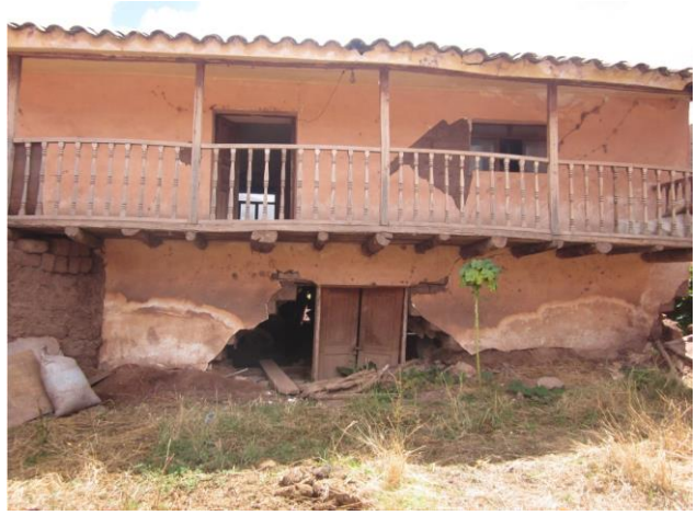
Figure 6-7: Home Affected by 2010 Cusco Floods (Source: Goshen College 2010)
