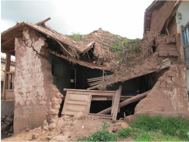
Figure 6-5: Home Affected by 2010 Cusco Floods (Source: Goshen College 2010)
