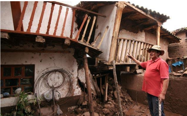
Figure 6-6: Homes Affected by 2013 Cusco Flood (Source: Cuatro casas 2013)
