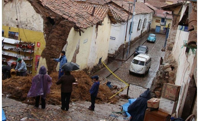
Figure 6-8: Homes Affected by 2013 Cusco Flood (Source: Cuatro casas 2013)
