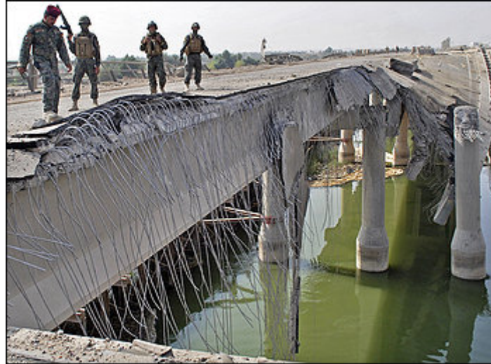
Figure 6.1: Bridge Destroyed in Iraq from Truck Bomb (The Washington Post, al-Mokhtar, 2009)
