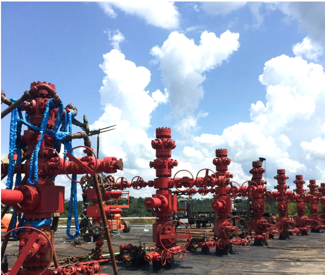
Figure 1.14. A hydraulic fracturing stack, composed of a series of high pressure components that protect the production wellhead during hydraulic fracturing operations. Source: Stock photography
