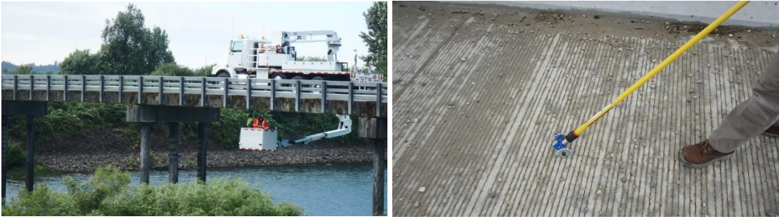
Figure 2: From [8] (left) visual inspection using snooper and (right) rotary impact tool to detect delamination
