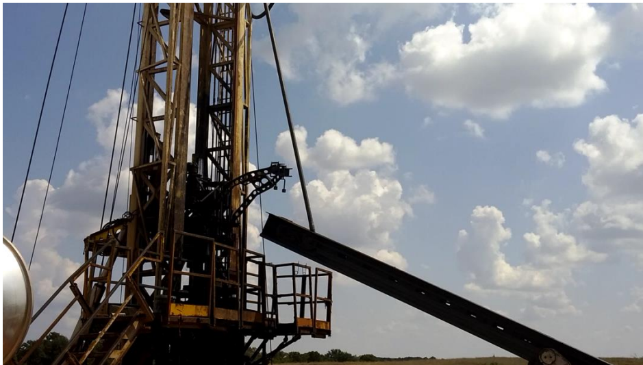
Figure 14. Catcher's mitt extended and ready to catch the new pipe coming from the catwalk.
