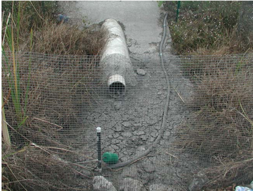
Figure 11 Photo of Modified Outlet (Trash Screen and Float Switch)
