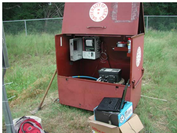
Figure 24 Outflow Sampler and Flow Meter
