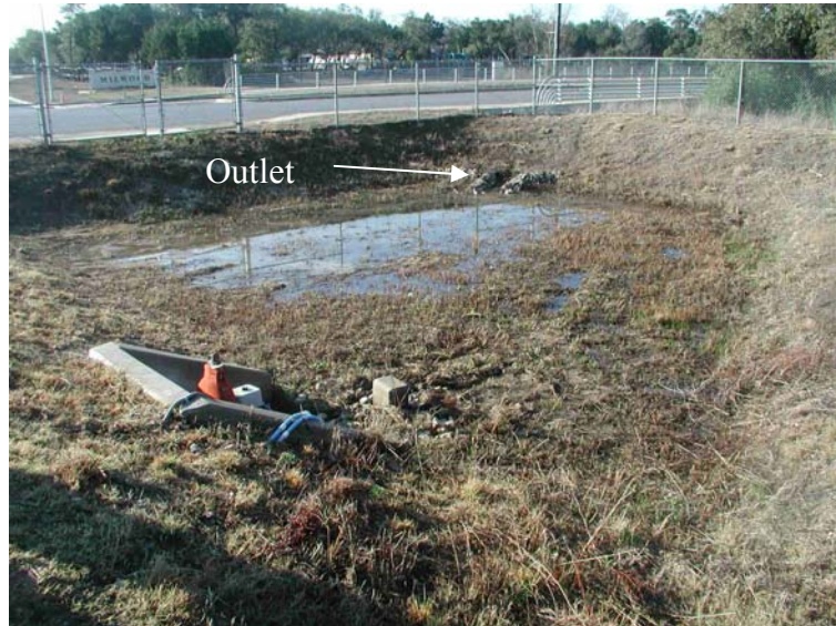
Figure 10 Photo of Modified Sand Filter Outlet Modifications
