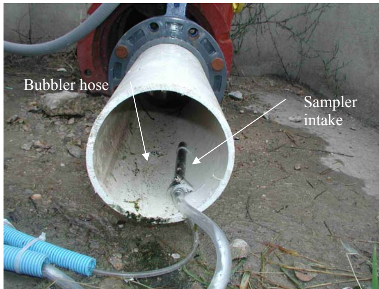
Figure 23 Outlet Sensor Placement
