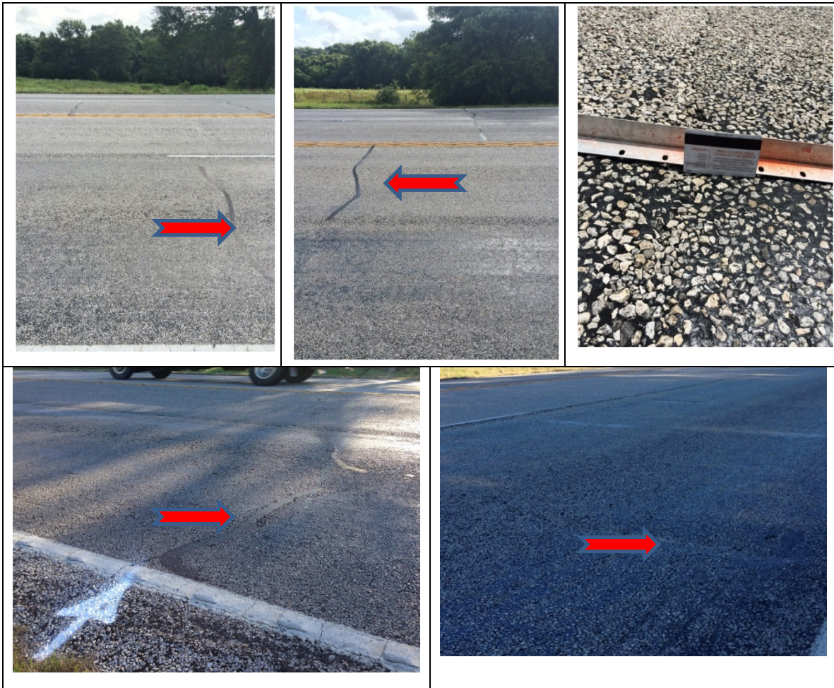
Figure 9: Images of transverse cracking along US77
