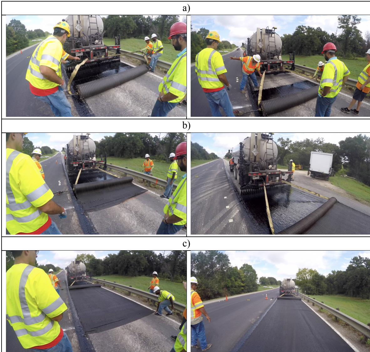
Figure 22: Interlayer installation sequence: a) looping tow strap through tack truck bumper and evening the strap; b) tack application and initial installment; c) continued installment and monitoring
