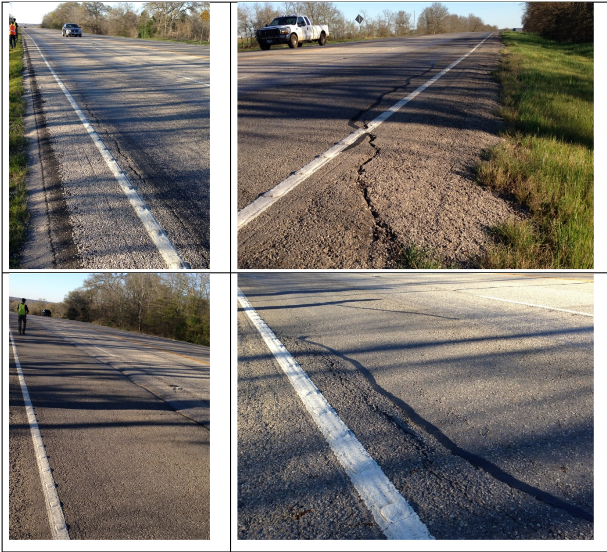
Figure 10: Images of longitudinal cracking along US77
