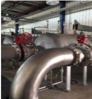
Figure 31 – Permeate pumps that lead freshwater to EPW's distribution system (Photo Credit: William Delgado-Thompson)
