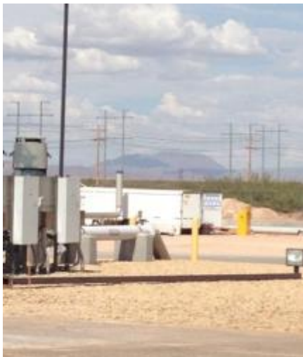
Figure 32 – Pipes that take concentrate to the injection wells (Photo Credit: William Delgado-Thompson)
