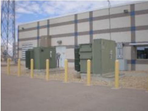
Figure 23 – The transformers that power the KBH desalination plant (Photo Credit: Art Ruiz)
