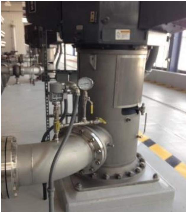
Figure 25 – High pressure feed pump that sends brackish water to membranes (Photo Credit: William Delgado-Thompson)
