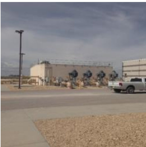
Figure 24 – Feed water pre-treatment facility (Photo Credit: William Delgado-Thompson)
