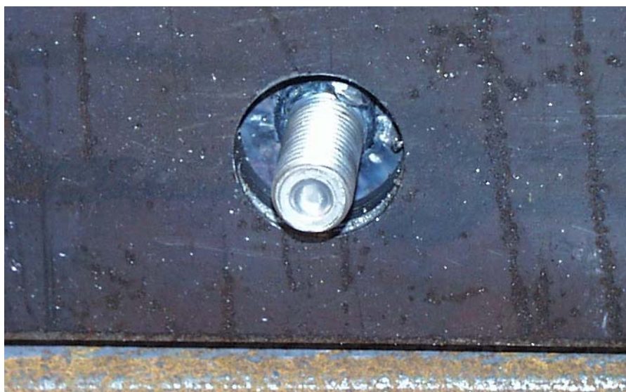
Figure 6.75 Gap around threaded stud
