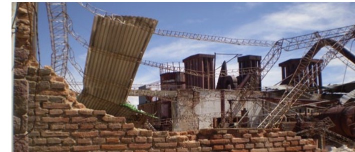
Remains of the Metal Huasi lead smelting plant in Abra Pampa. Photo by Jessica Osorio.
