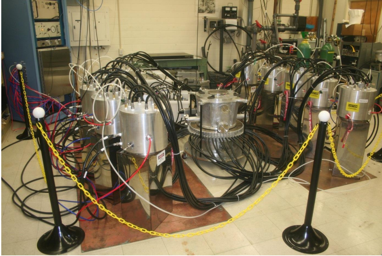
Figure 3.3 The completed 10 capacitor system at UT, showing all the cables and switch can assemblies connected to the target chamber. The control rack is in the background on the left. This setup was used to test the system for magnetic field production.
