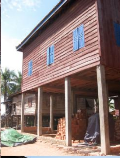
Photo 5: A home in progress, representing the typical piecemeal construction strategy that migrant households use to construct an ideal home over time.
