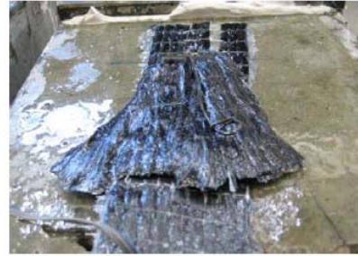
c) Debonding of CFRP anchor
