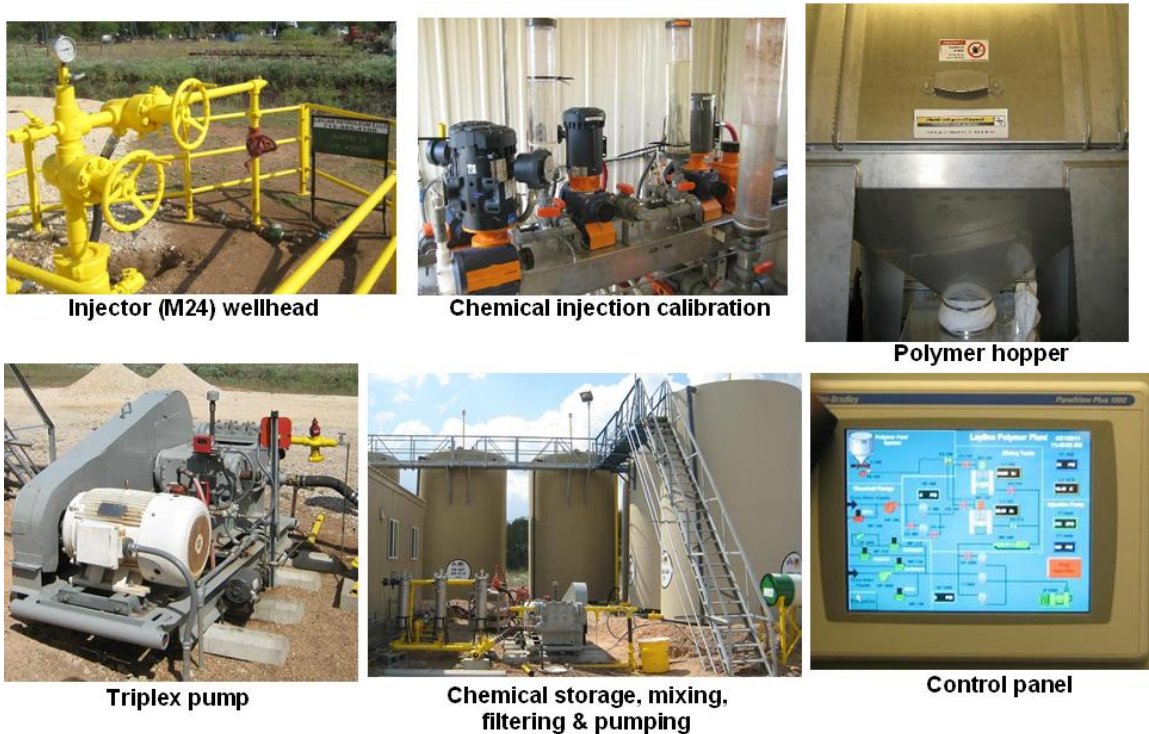
Figure 10.1 Surface Facilities Installed at Pilot Location.
