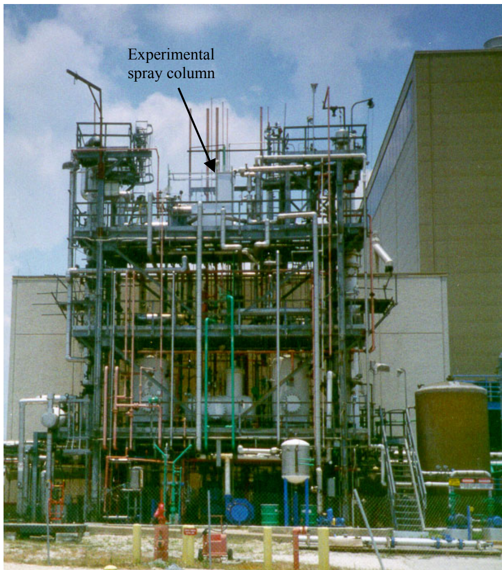
Figure D.1. Pilot facility of the UT Separations Research Program
